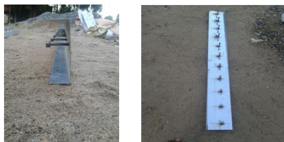
Figure 6.1 Cold form steel with shear connectors Corrosion treated cold formed steel trough section was placed on a level floor, core reinforcing system was kept above with minimum cover and then concrete was poured
